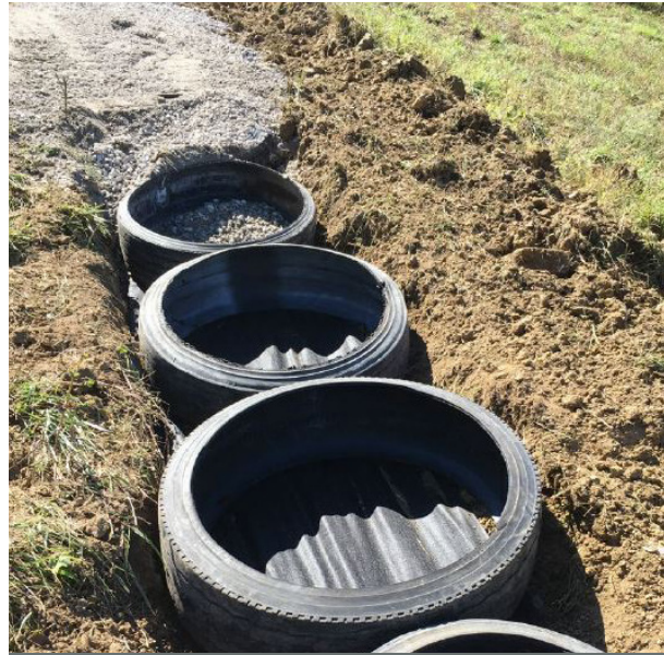
Nonwoven geotextile fabric and tread cylinders are placed in a trench and backfilled with dense grade aggregate (DGA).
